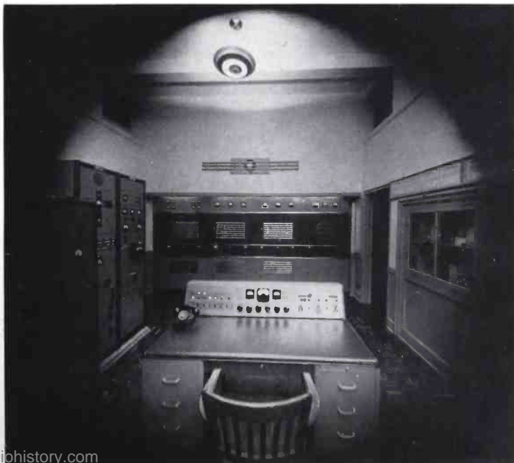
FIG. 1. 5-DX transmitter at WSYR, Syracuse. Cabinet for spare tubes and components is at the right; monitoring equipment and emergency transmitter at the left.
