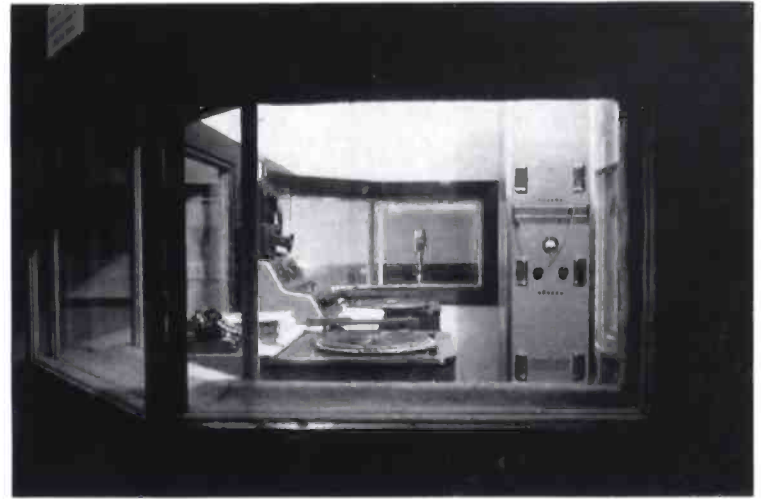
FIG. 4. Control room for two of the smaller studios of Radio Nacional, Rio de Janeiro. (See also Page 28.)
